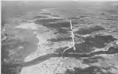
CUTTING THROUGH the heart of the cunucu is the roadbed for the new highway. PASANDO DOOR di curazon di cunucu ta e carretera nobo bajo construcion.
